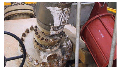
Competitor's valve leaked acidic slurry.
